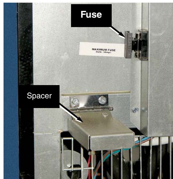
Fuse Box and Cover
